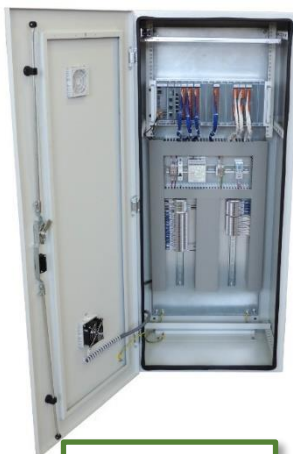
Example of cabinet for smaller substation
